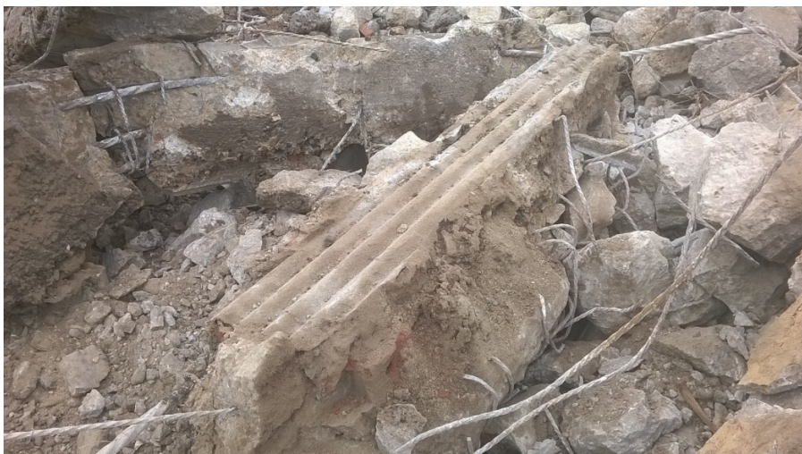
Photograph 01 - view of the chrysotile cement board surrounding a ground beam. Photograph provided by Brims Construction Limited.
